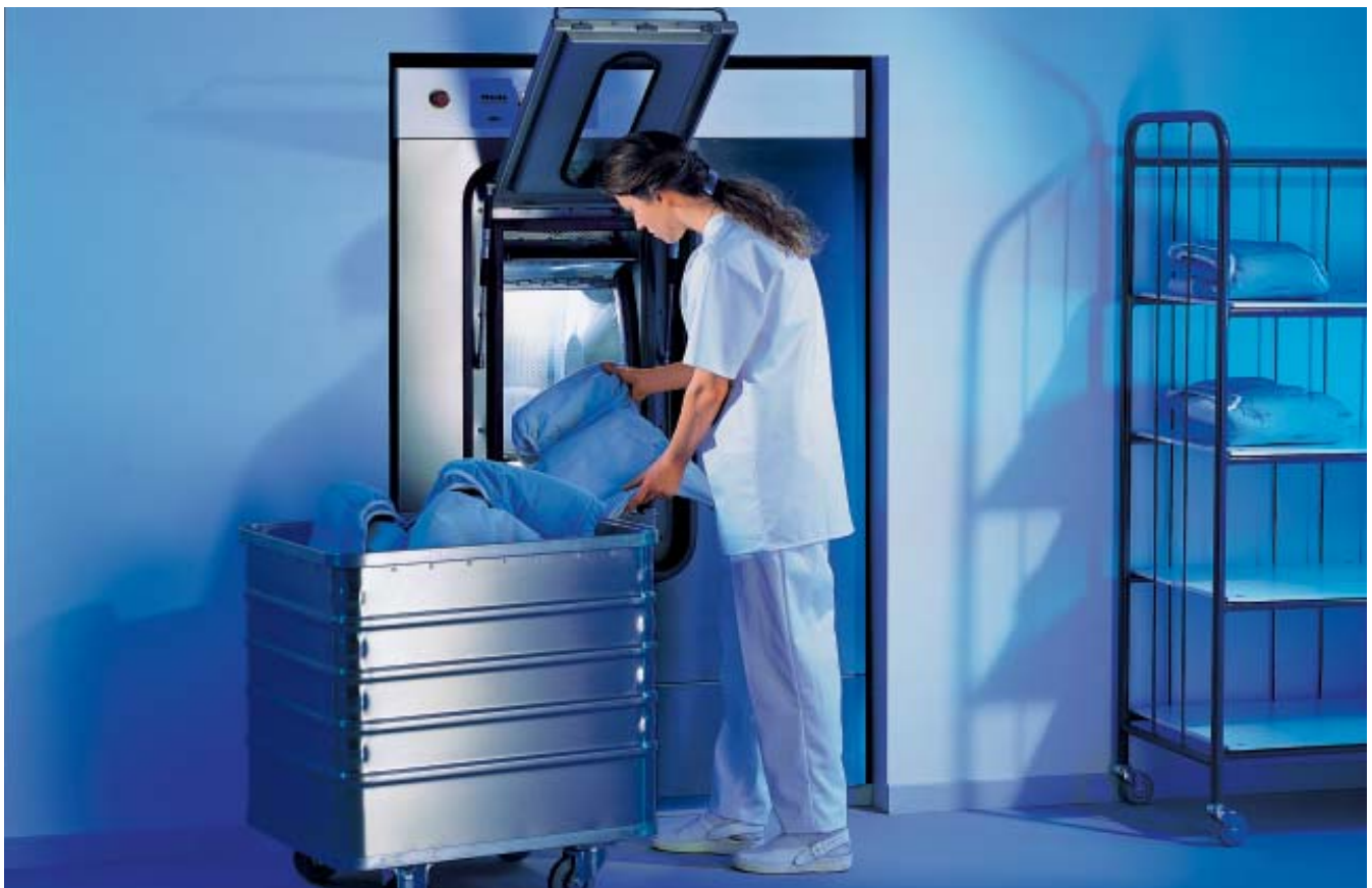
Clean side: Unloading a machine installed into a dividing wall
